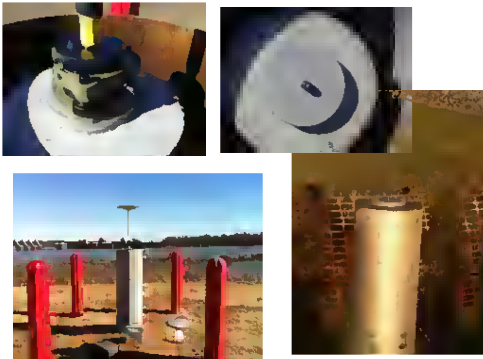
Figure 2-7. Reference point monumentation. Concrete pier construction vicinity of a lock and dam. Forced centering plug set into concrete pier. (Little Rock District).
